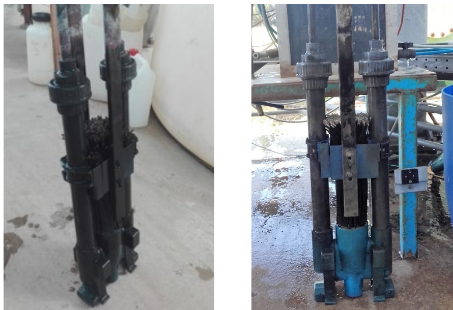
Figure 3-11. Hollow-fiber membrane module before (left) and after (right) the chemical cleaning.
