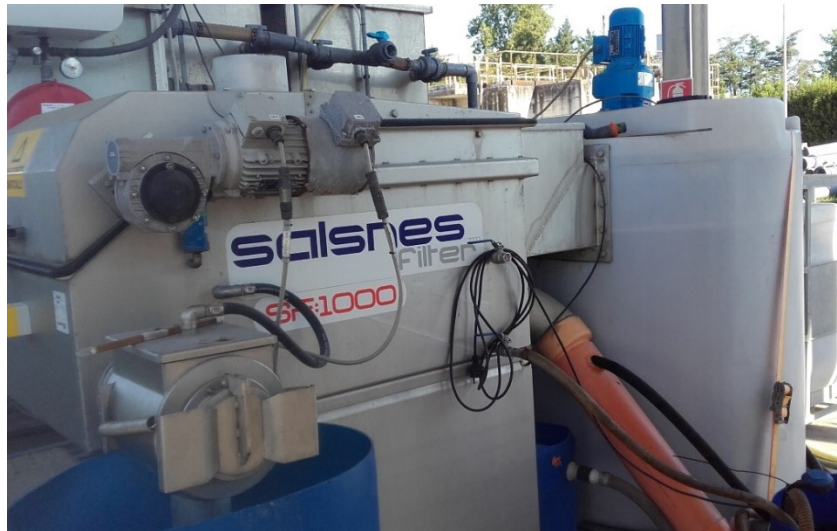
Figure 3-10. Salsnes Filter used as primary treatment in the second and third configuration.
