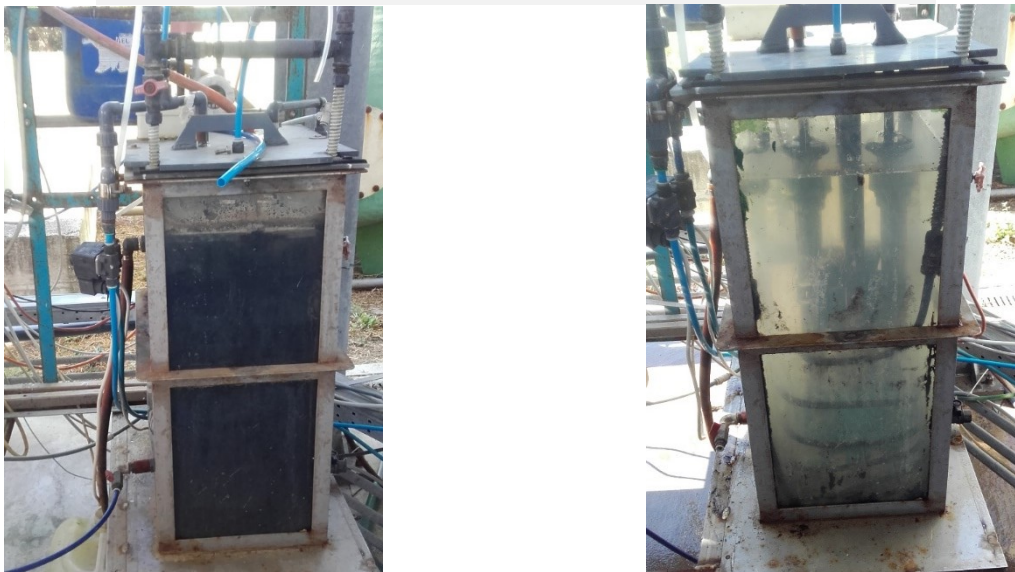
Figure 3-9. Anaerobic Membrane Reactor during operation phase (left) and after maintenance cleaning (right)
