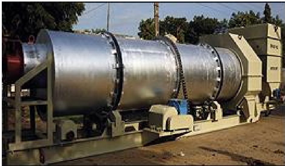
Figure 8. Dryer-drum in Asphalt Plant (Sit.2).
