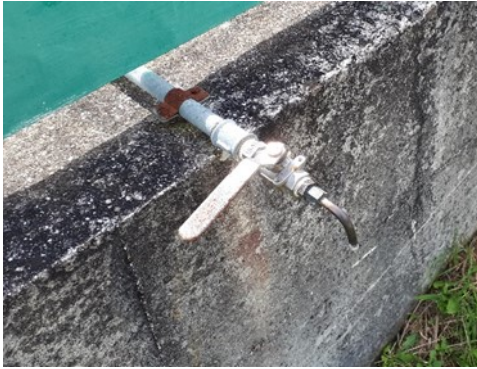
Figure 24 Intake at drinking water plant inlet (1)
