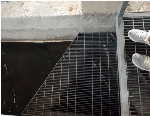
Figure 29 Inlet to filtration sampling point
