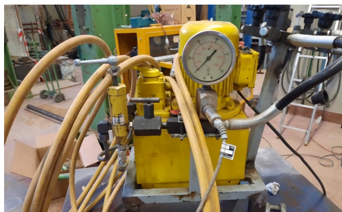
Fig.29 – Centralino Enerpac (Fullbridge)
