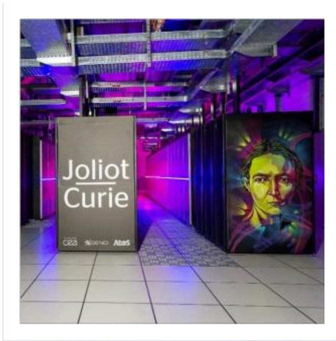
Fig.14: n Joliot-Curie IRENE-KNL supercomputer in CEA's Very Large Computing Centre (TGCC)
