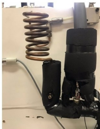
Fig. 2.10 – Serpentina in rame esterna
