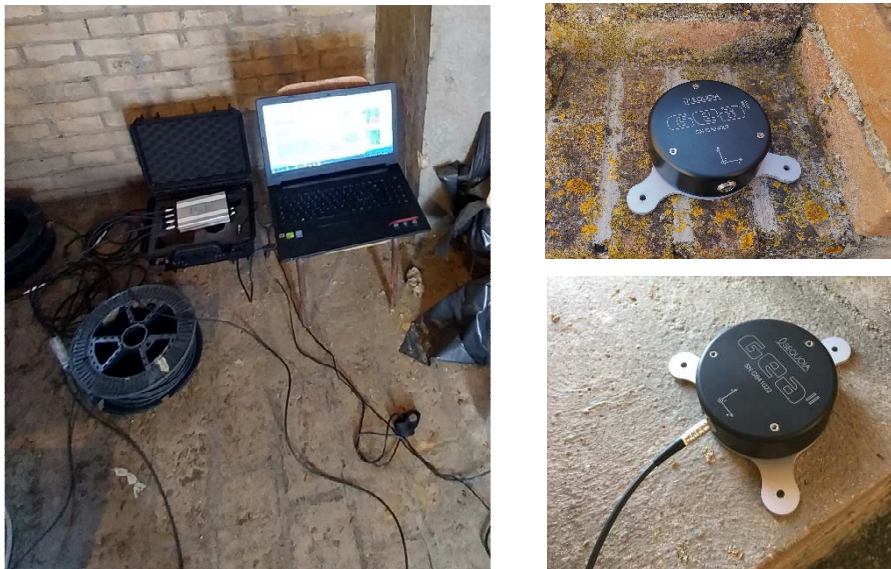
Figure 3-2 – On the left, a photo of the central processor; on the right, two pictures of the positioning of the sensors
