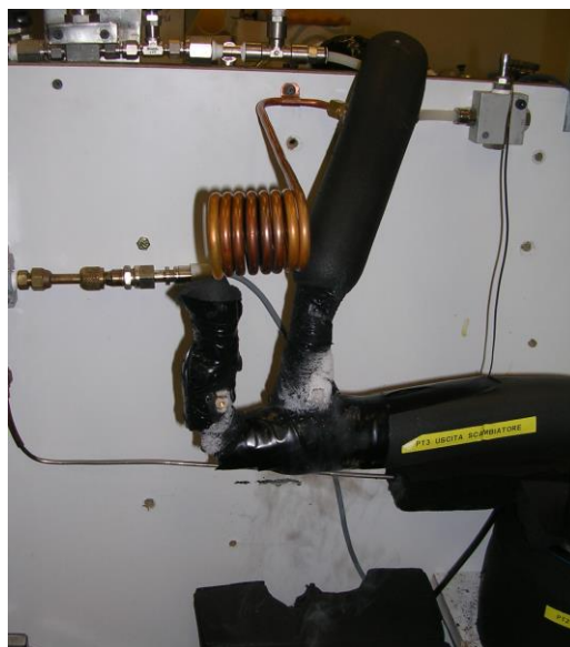
Fig. 3.11 – Serpentina in rame esterna
