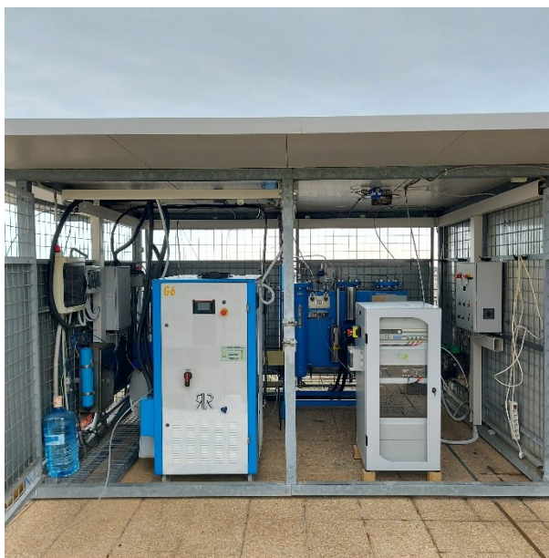
Figure 26 – Alkaline electrolyzer installed at DIISM [18]
