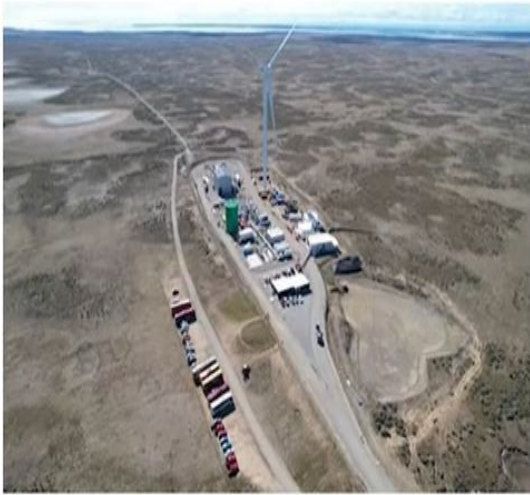
Porsche, "Haru Oni" pilot plant Punta Arenas (Chile) From: Porsche Newsroom, December 20 th , 2022
