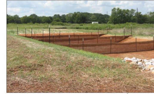
Figure SBN-3: Example of porous baffle made of 700 g/m 2 coir erosion blanket as viewed from the inlet
