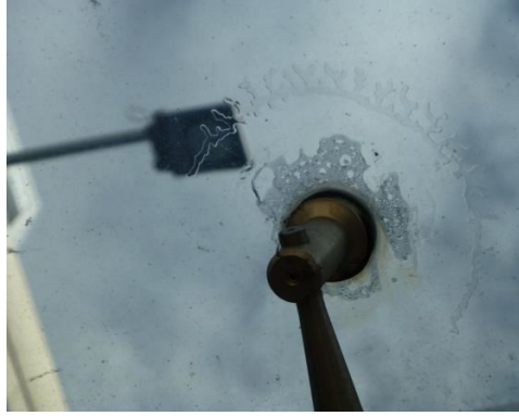
Figure 4.9 Delamination phenomenon around a parapet hole
