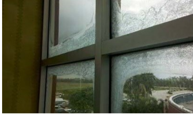
Figure 4.10 Delamination in an Insulated Glass Unit
