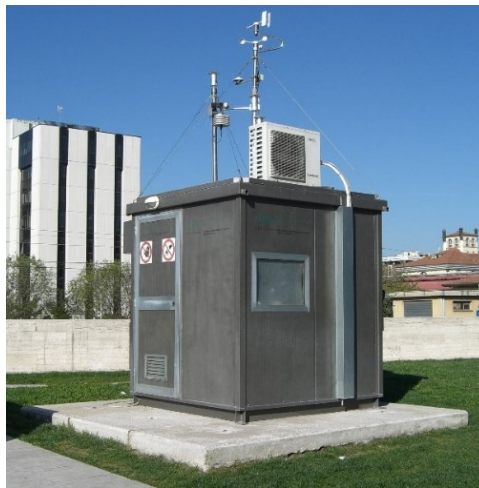
Fig. 1.1 – Air quality monitoring station
