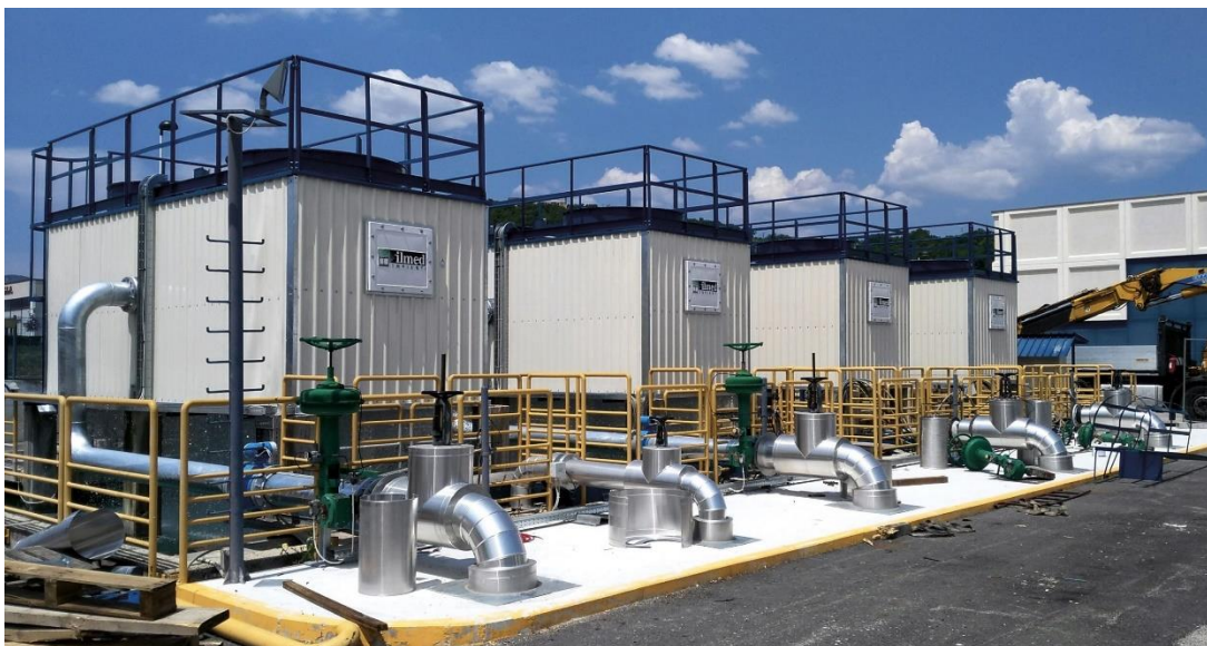
Figure 42: ILMED cooling tower system
