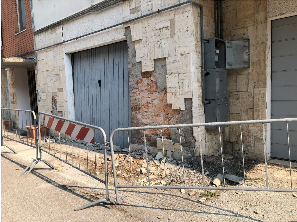
Figure 2. Effects of land subsidence processes on the buildings of the Madonnetta district of Pioraco, July 2022.
