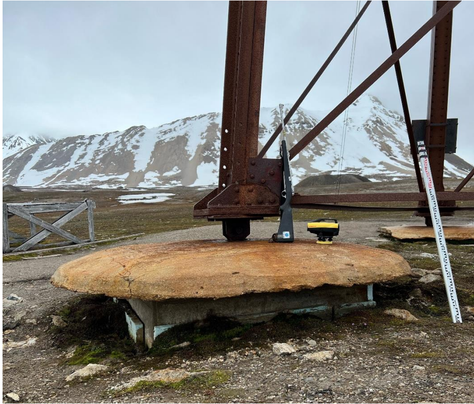
Figure 10.8 Luftskipsmasta, visible permafrost degradation under the foundation concrete place.
