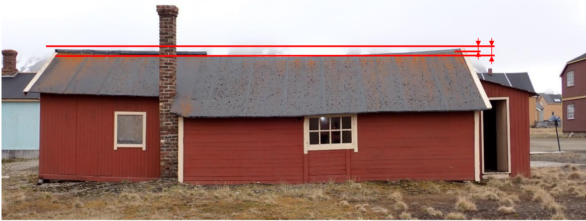
Figure 10.6 Green Harbour House settlement of ca. 15 cm already visible from field investigation. Wooden foundations decay must be expected.
