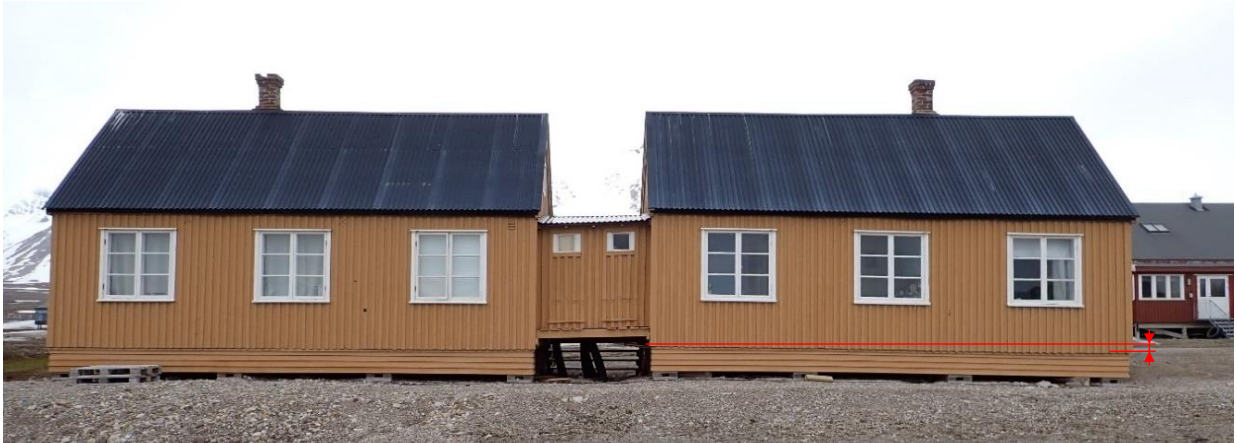
Figure 10.7 London Houses settlement of ca. 12 cm already visible from field investigation.
