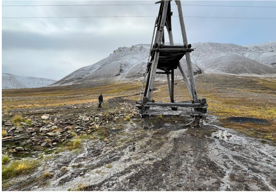
Figure 6.10 Rock and land-slide adjacent to the structure and stream flowing at the base of the structure.
