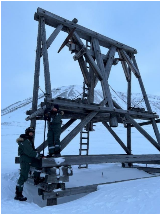
Figure 6.9 Small structure settlement and displacement
