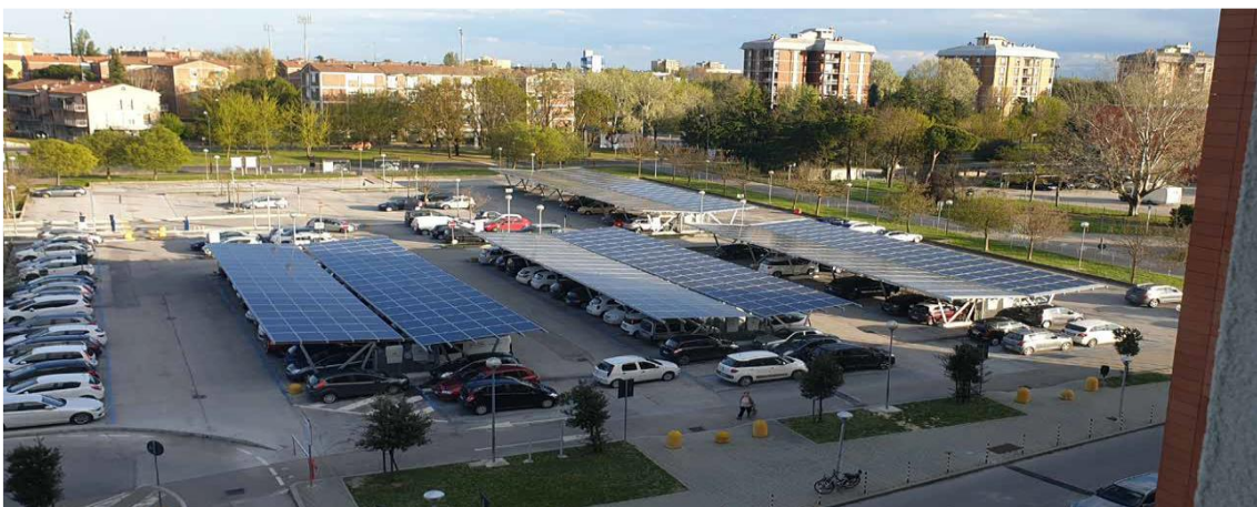
Figure 8: Example of a carport installed in a parking area.
