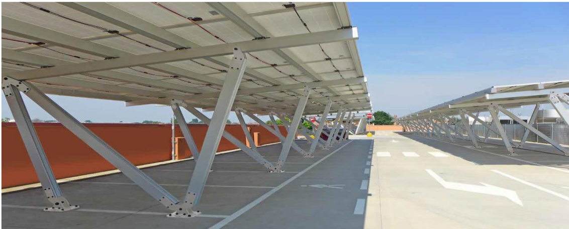
Figure 7: Example of a carport installed in a parking area.
