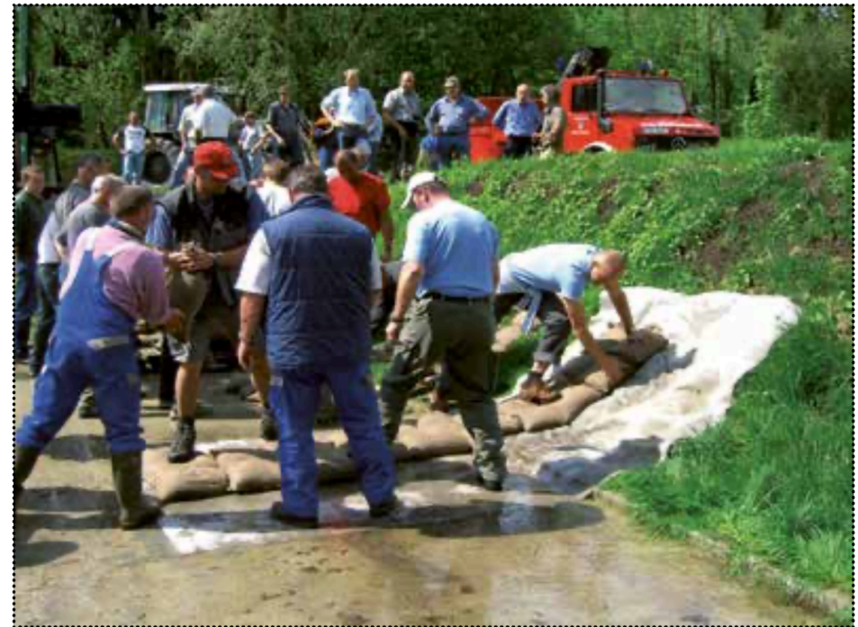
Figure 5 – Dyke defence: Exercise course on the fire brigade training ground in Rosenheim. (State Office for Water Management Rosenheim)
